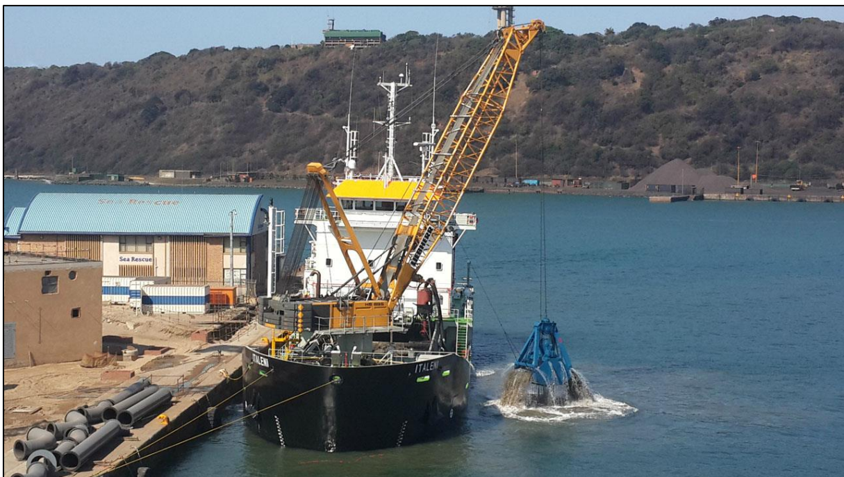
Figure 12-1: Self-propelled grab hopper dredge.
