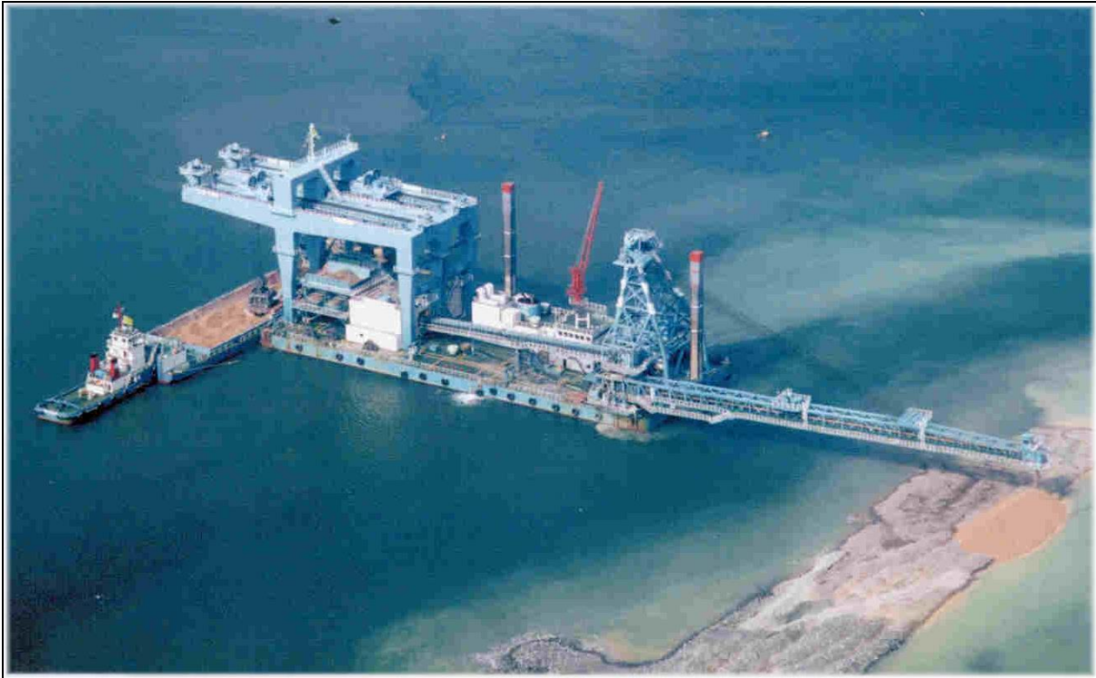
Figure 12-2: Grab bucket reclaimer.
