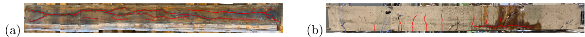
Fig. 4. Pictures of the crack patterns (a) after corrosion of beam U in bottom view and (b) after sustaining a 48 kN load during four-point bending of beam L_{sym} in side view.
