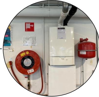
Gas boiler heating (space heating & hot water)
