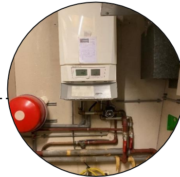
Gas boiler heating (space heating & hot water)
