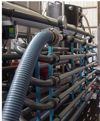
Figure 2.12: Photograph of the tube flocculator, which is used in some of the pilot investigations
