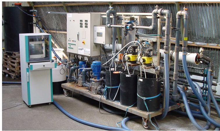
Figure 2.7: Photograph of the pilot ultrafiltration installation
