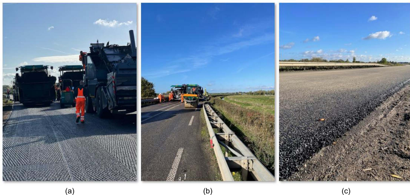
Fig. 1. (a and b) View of paving operations; and (c) compacted test section at N837, Province of Gelderland, the Netherlands.
