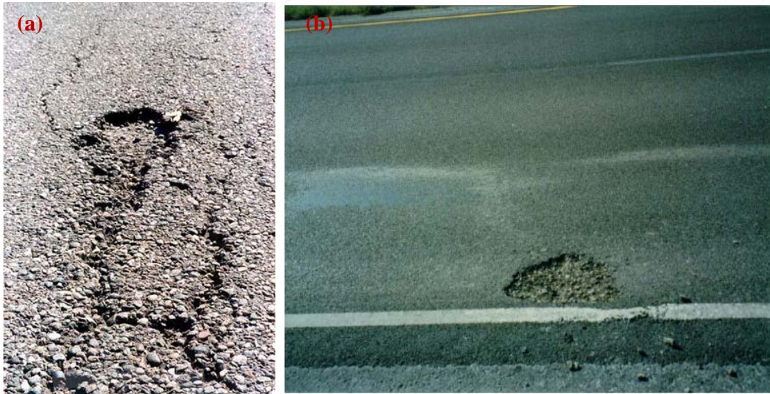
Figure 1.1 Deteriorated pavements due to water induced damage: (a) ravelling caused by segregation and (b) potholes caused due to stripping Reprinted from Pavement Interactive ( http://www.pavementinteractive.org/ ).
