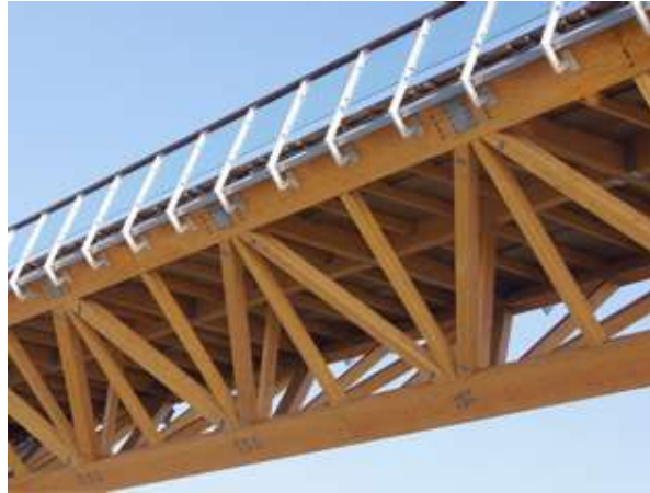
Figure 4.52: Complex node in the Anaklia-Ganmukhuri bridge using slotted in steel plates and the HESS Limitless joint for the splice joint of the inner ring
