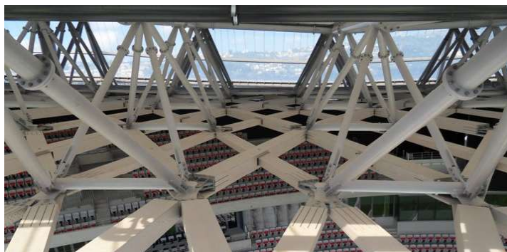
Figure 2.30: Detail view of the spaceframe of the Allianz Riviera stadium in Nice
