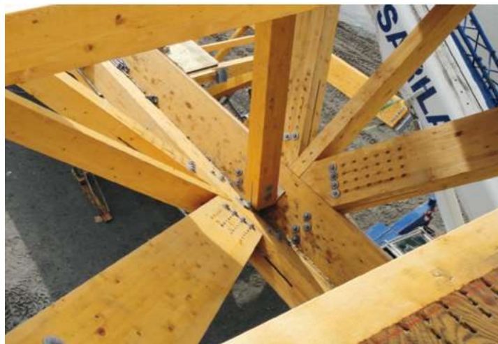
Figure 4.49: Complex node in the Anaklia-Ganmukhuri bridge for the internal connections of the outer truss ring
