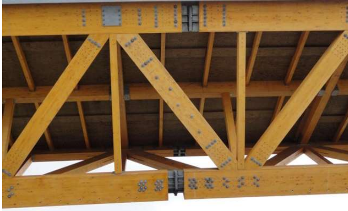
Figure 4.50: Complex node in the Anaklia-Ganmukhuri bridge using cast steel parts for the splice joints in the outer truss ring
