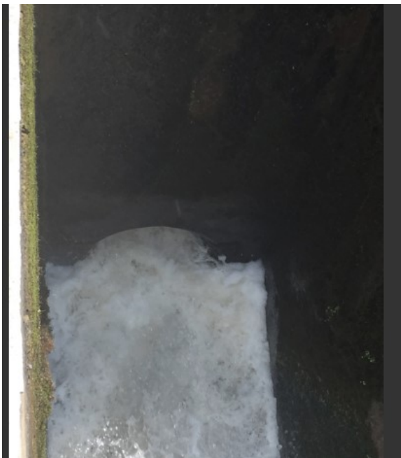
(a) air intake pipeline
