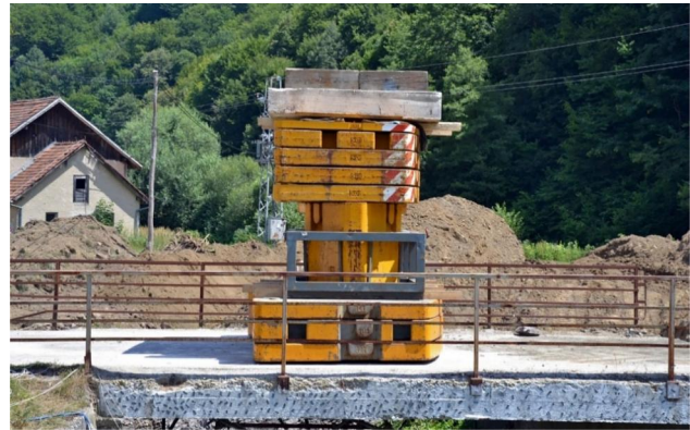
Figure 12. A proof-load test following a SLT on a test bridge in Slovenia.
