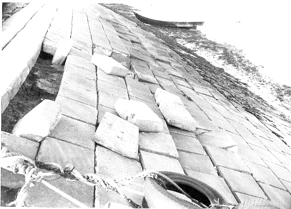
Fig. 163. Damage to a berm (tapered blocks).
