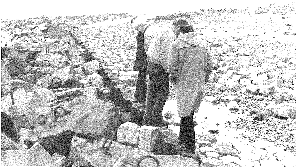
Fig. 172. Damage to the Maasvlakte south wall (the rubble layer on the toe is to the left, the remains of the revetment are to the right).
