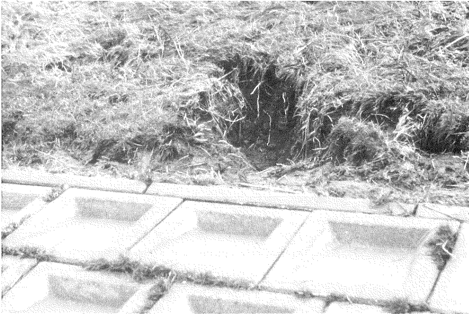
Fig. 74. Erosion of grass above the revetment.
