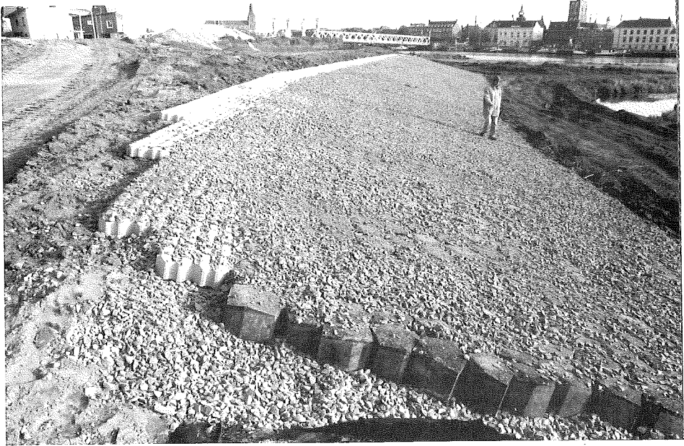
Fig. 13. Washed-in concrete columns on a thin filter on top of a geotextile. Four rows of “growth” blocks are placed along the upper edge of the geotextile.
