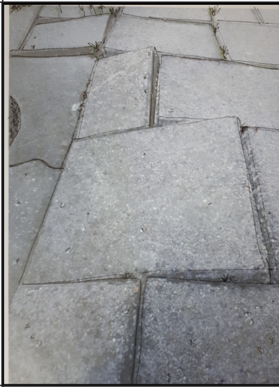
Loose tiles are not comfortable.
