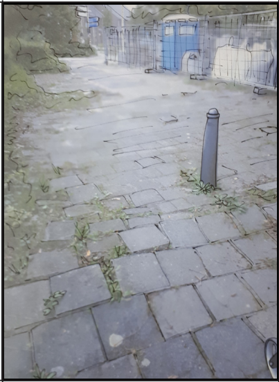
The loose tiles are difficult to walk on.
