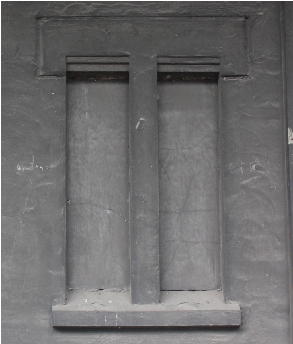
Fig. 98. Current state of the windows in the facade of Katoenveem, source: photograph by C. de Boon
