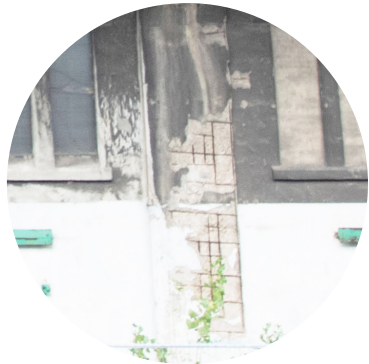
1. Corrosion of the reinforcement
