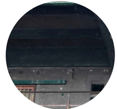
9. Black surface, deposit of soot
