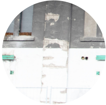
2. Spalling of render layer and concrete layer
