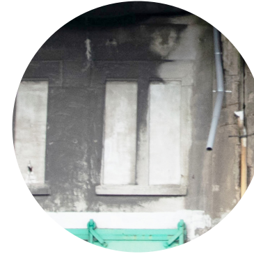
6. Closed off or broken windows
