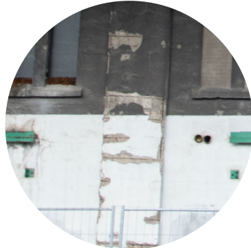
2. Spalling of render layer and concrete layer
