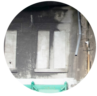
6. Closed off or broken windows
