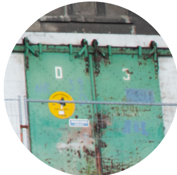
4. Corrosion of original sliding doors
