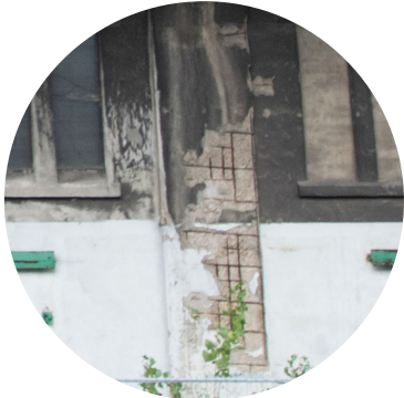
1. Corrosion of the reinforcement
