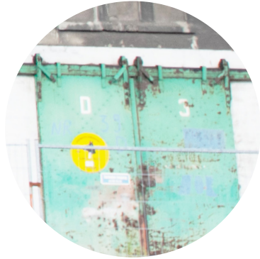
4. Corrosion of original sliding doors
