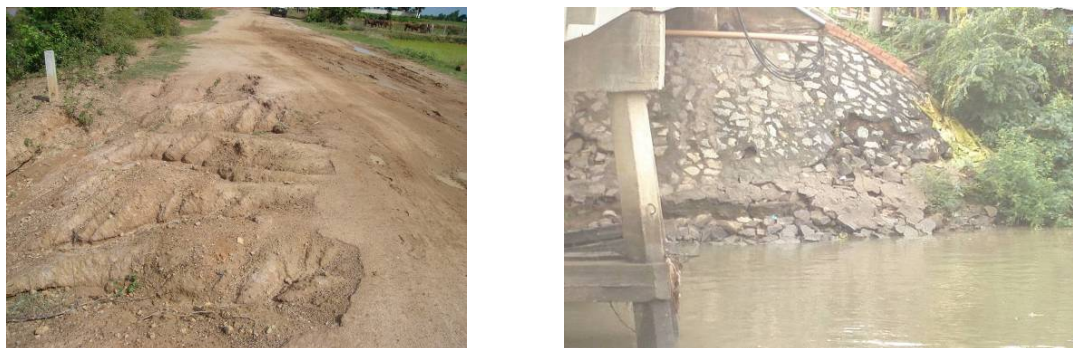
Figure 2.4 Examples of damage due to floods; damage to an unpaved road (left) and damage to a bridge abutment (right).
