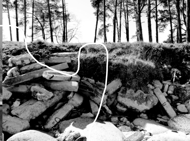
Response to coastal erosion
