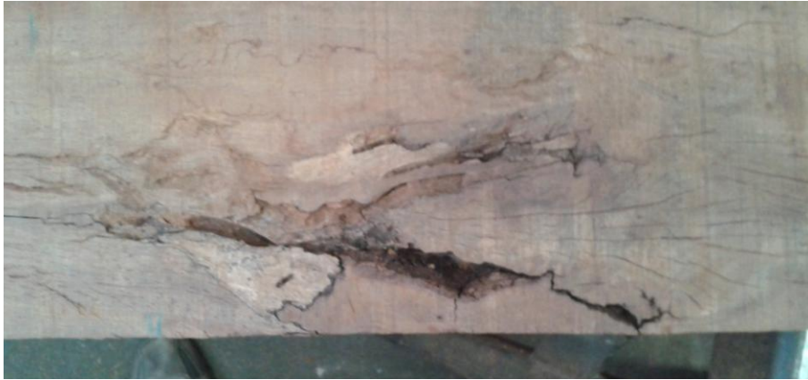
Figure 3.11. Anomaly in a timber beam that might affect the strength in an unpredictable way. Timber with these kinds of anomalies should not be used as structural timber
