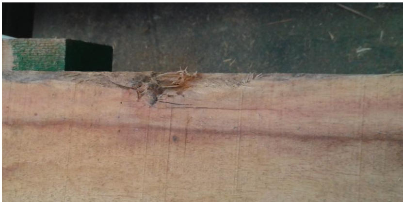
Figure 3.10. Wane in a timber beam.
