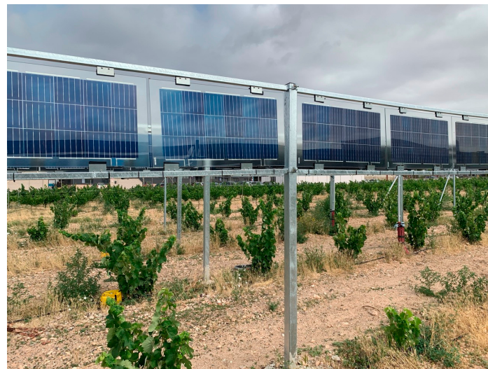
Figure 2. Vertical bifacial pilot installation.
