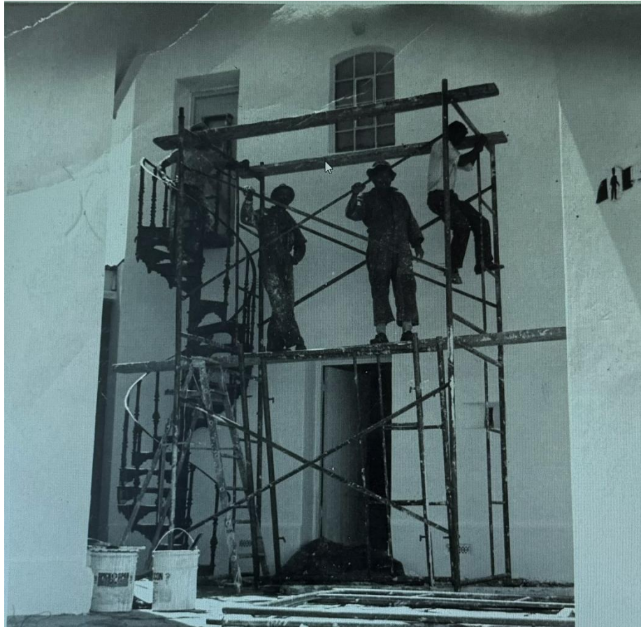
Figure 3: Alte Feste, Windhoek, renovation work, original photographer and date unknown, National Archives of Namibia.
