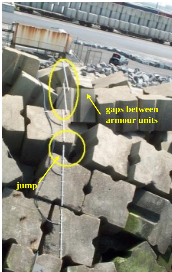
Figure 4.33: Indication of blocks sticking out of the mean slope and gaps between two neighbouring armour units.
