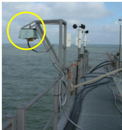
Figure 4.10: Infra red meter installed on the measuring jetty.
