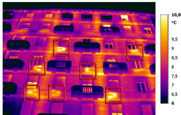
Figure 8 - Detail of the temperature distribution on the upper part of the façade (Case Study 2), above the main entrance. In the red squares, the warmer areas due to the heat flux generated by the heaters. The reduced thickness of the masonry where the heaters are located causes higher surface temperatures, especially at the connections between the heater and the hot water pipes.
