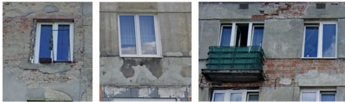
Fig. 6 Examples of deterioration, Grochowska 271, 275, 283. (Google Street View, 2024)
