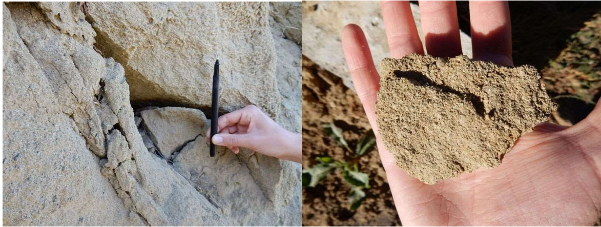
Figure K-3: Close-up of slope material showing opened up joints (left) and medium-grained texture of rock (right)
