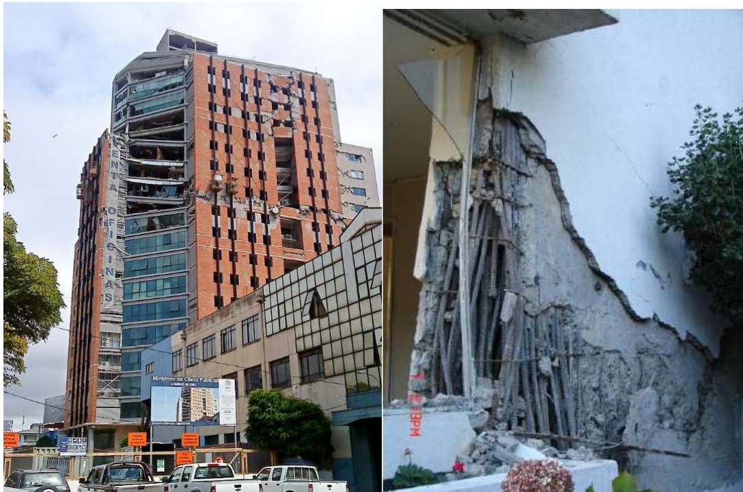
Figure A-10: (Left) Partially collapsed O'Higgins Tower, Concepción; (Right) Damage to typical unconfined shear wall boundary zone observed in Concepción (ASCE 2010)
