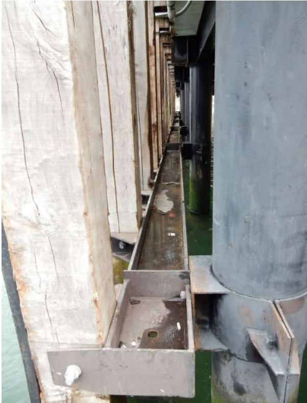
Figure C-9: Connection steel piles to wooden fender with rubber strip to absorb kinetic energy of vessel
