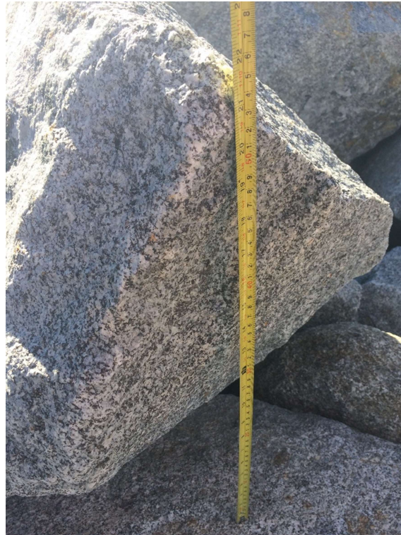
Figure I-2: Close-up of granitic armourstone used for shore protection rubble mount at Dichato
