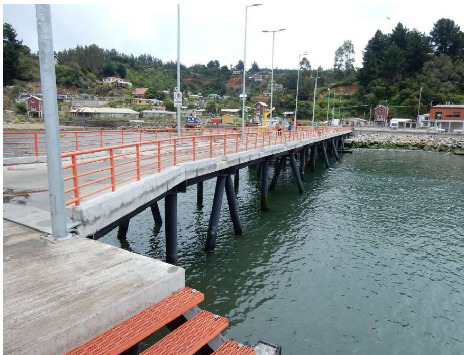
Figure C-6: Jetty with concrete deck and steel piles, some battered to resist lateral loads
