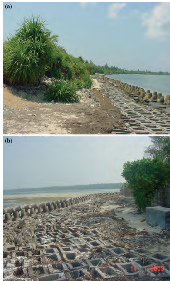
Figure 3. Coastal protection measures along the coast of Lakshadweep with hollow concrete blocks and tetrapods
