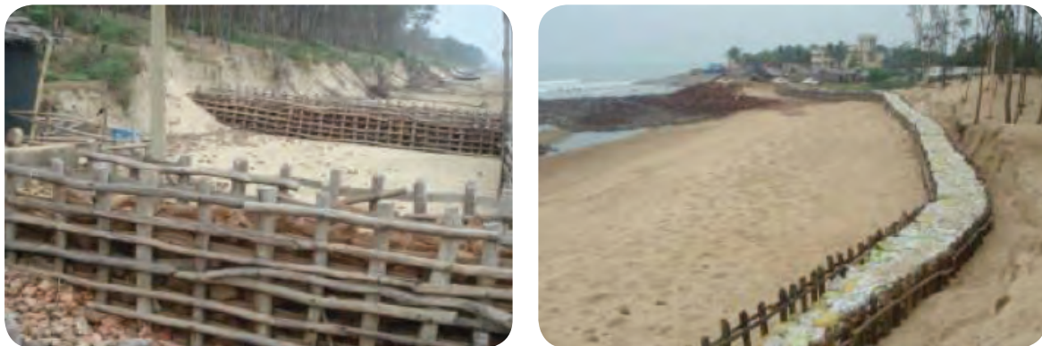
Figure 14. Erosion scarp on the frontal dune and temporary protection at Digha, West Bengal. The old dunes are seen behind the coastal works
