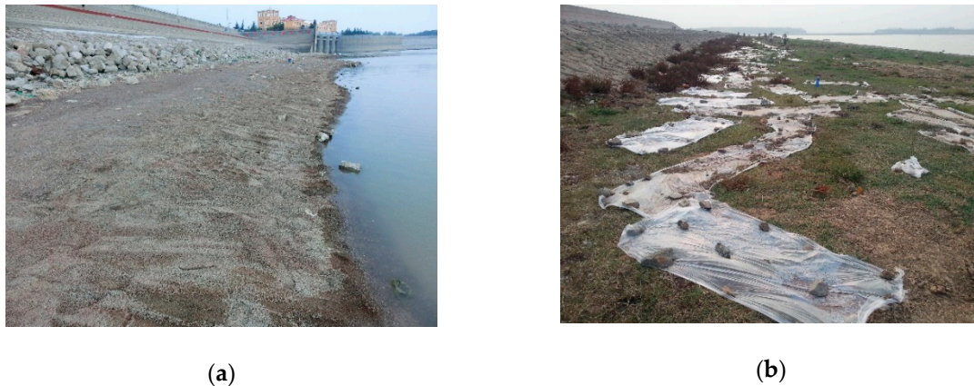
Figure 5. Treatment and prevention measures for cracks on the upstream slope of the dam. (a) Cover with stone flour; (b) Moisture retention with plastic sheets.
