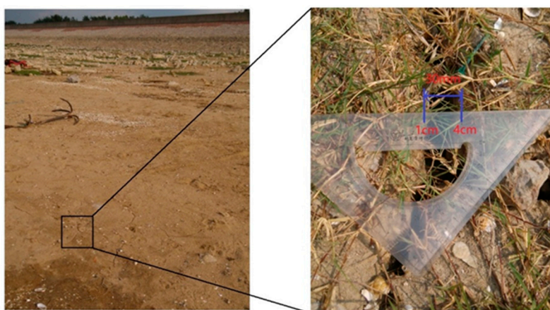
Figure 4. Cracks with maximum width of 30 mm on the upstream slope.
