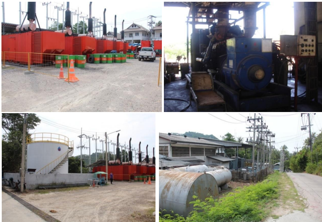
Figure 18: Generators and diesel tanks at the government owned power plant
