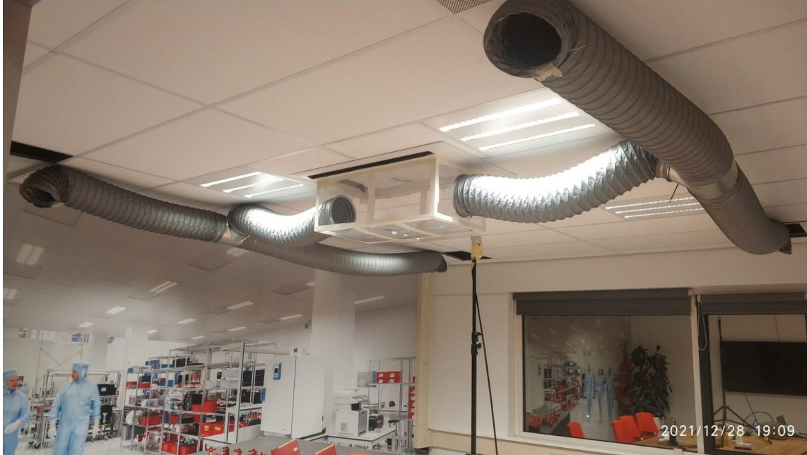
Figure 65 the draft ventilation renovation product model (photo from author)
