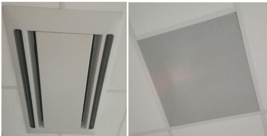
a) indoor end unit ceiling surface.
