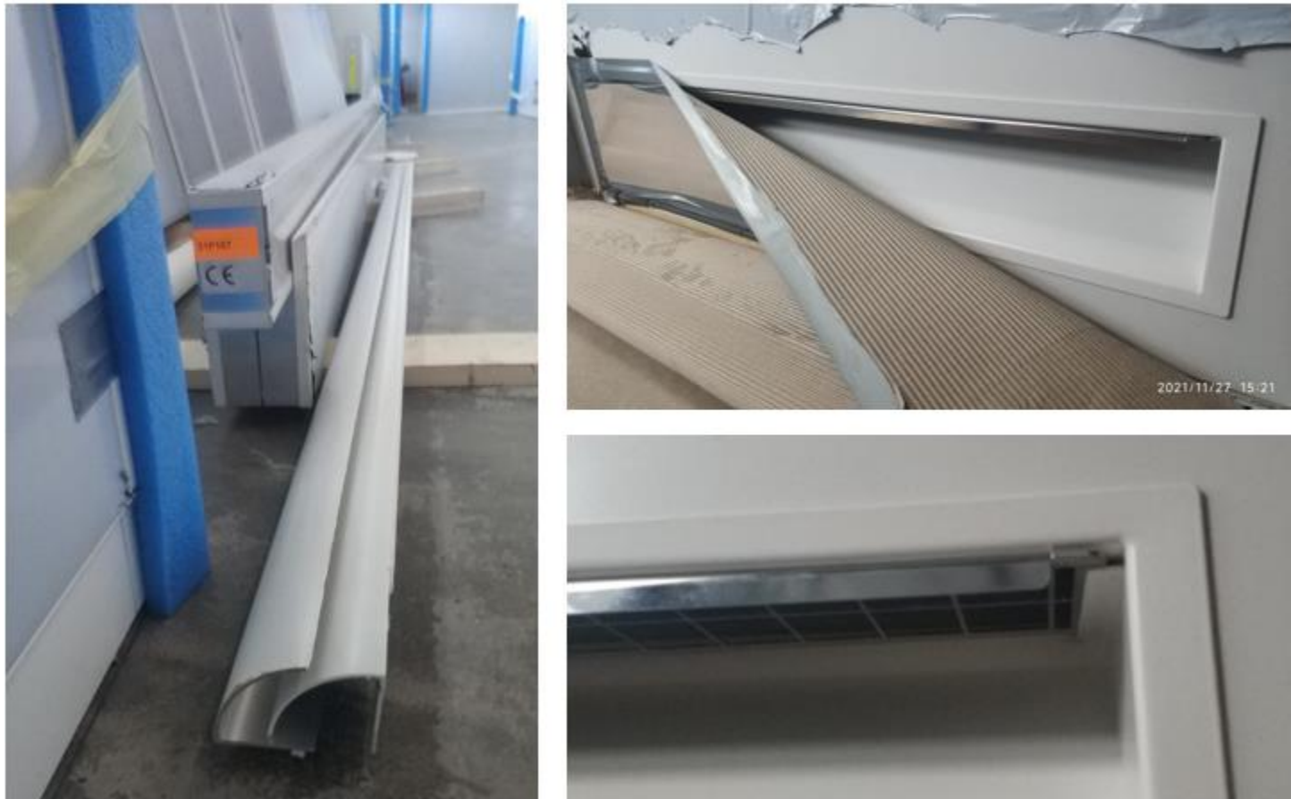
Figure 47 The construction site of cleanroom ventilation system installation from Kuijpers (photo by the author)
