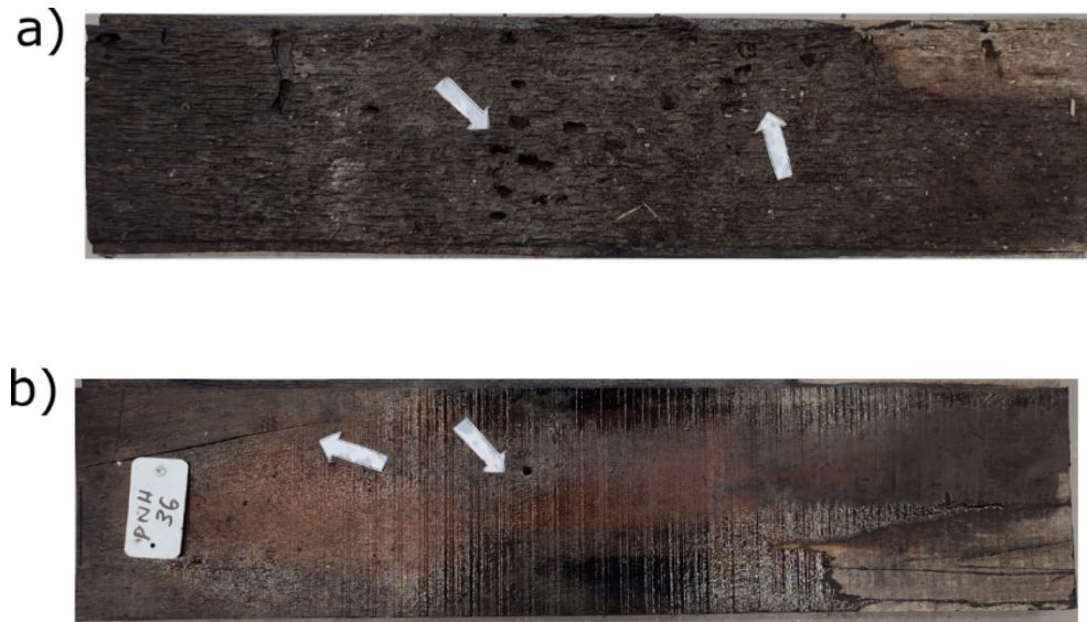
Fig. 2 Detrimentation on water side (a) and earth side (b), with arrows highlighting the holes due to marine borer attack
