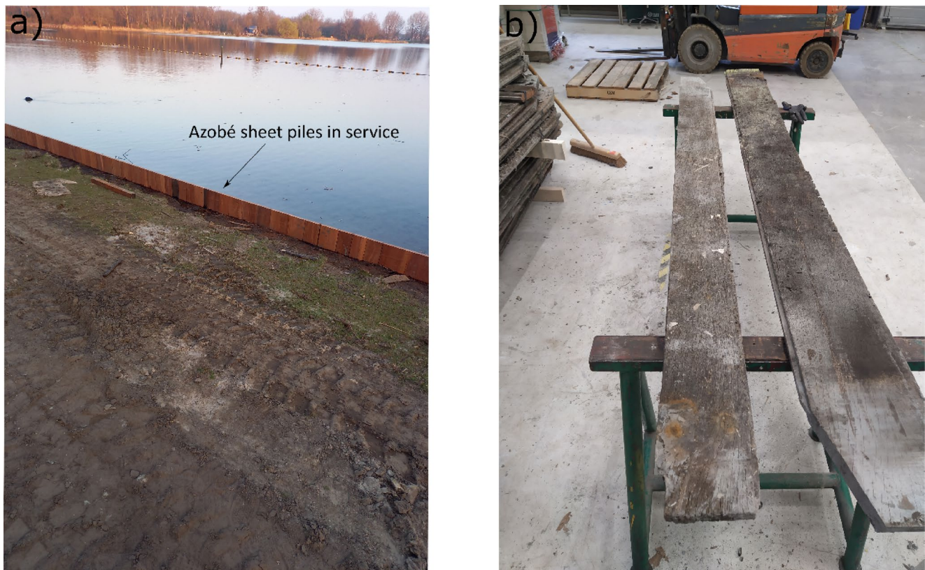
Fig. 1 Full size azobé sheet piles (a) in service at Delftse hout, Delft, The Netherlands; (b) pulled out after 57 years of service from Medemblik, the Netherlands
