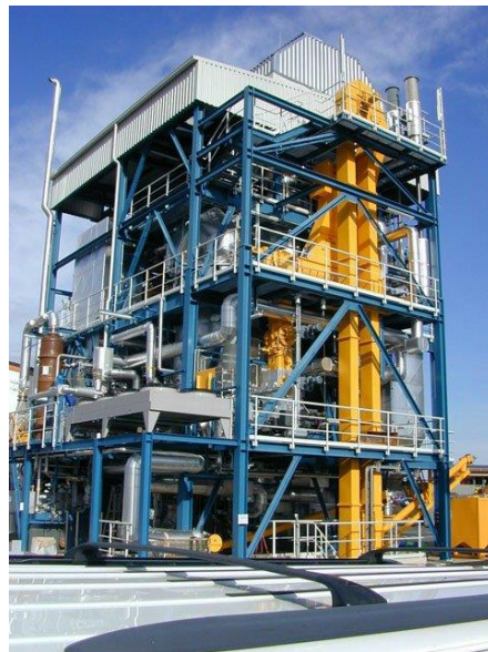
Figure 37 Biomass CHP Plant Güssing (AER, 2007)
