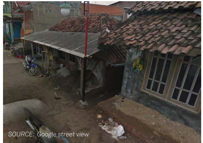
House subsiding, but with floor raised
