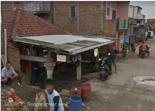
House subsiding, but with floor raised
