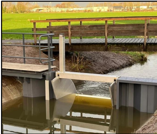
Figure 6 - An automated adjustable tilt weir with an RTC box (top right), which monitors the water level at the weir by automatically processing incoming data and adjusting the weir as needed to maintain a set point of a certain water level height. Picture from GWW-Bouw .
