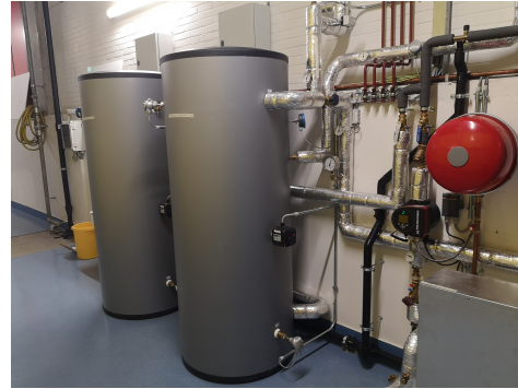
(b) Two 500L water tank
