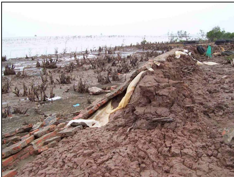
Figure 5.4 Breached dyke of shrimp farm, built of clay and trees
