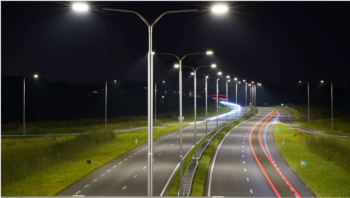
Figure 22 N279 road light in North Brabant
