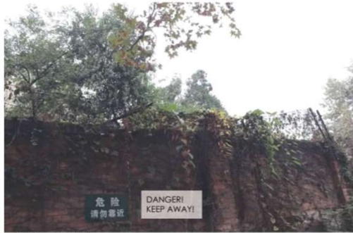
Aging dangerous wall.
