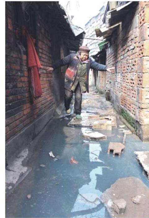
Aging drainage system.
