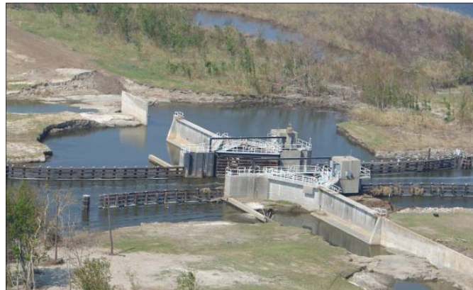
Figure A-4: The transition suffered from extensive erosion due to overtopping (picture: Les Harder)
