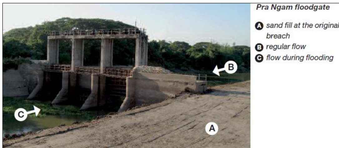
Figure A-6: Failure next to the Pra Ngam floodgate
