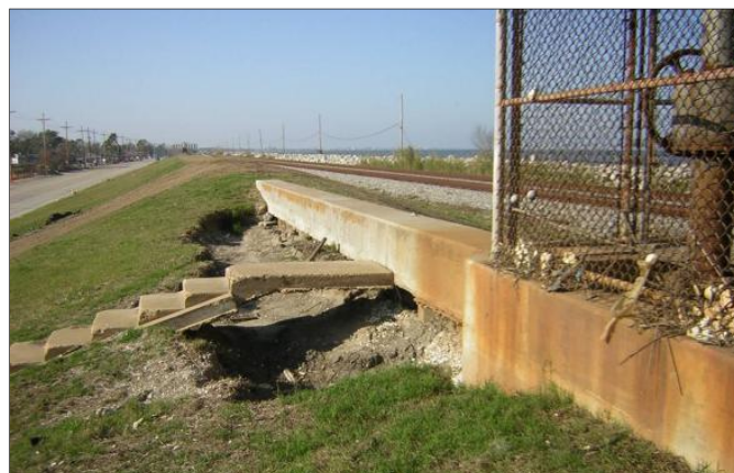
Figure A-2: Observed scour at a pump station structure transition with soil (picture: Rune Storesund)
