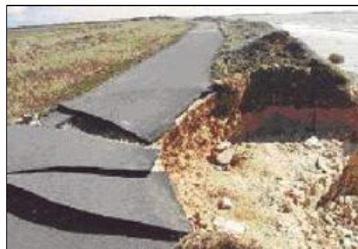
Figure A-5: Failure at the transition between an earthen structure and a promenade (Kolen et al., 2010)
