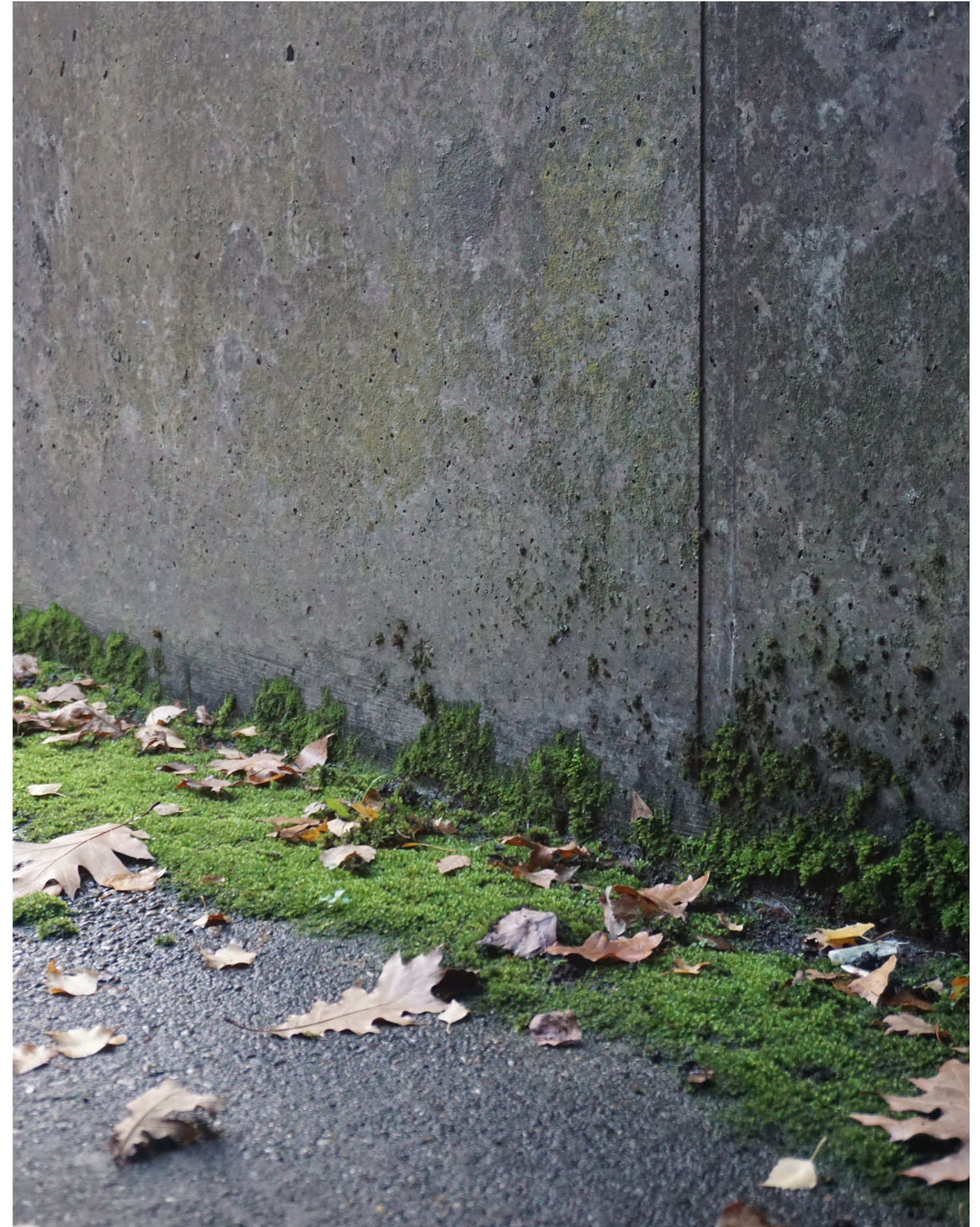
Figure 59. Moss growing on the concrete shell of the rear of an air shelter at ASA. Source: Own work.
