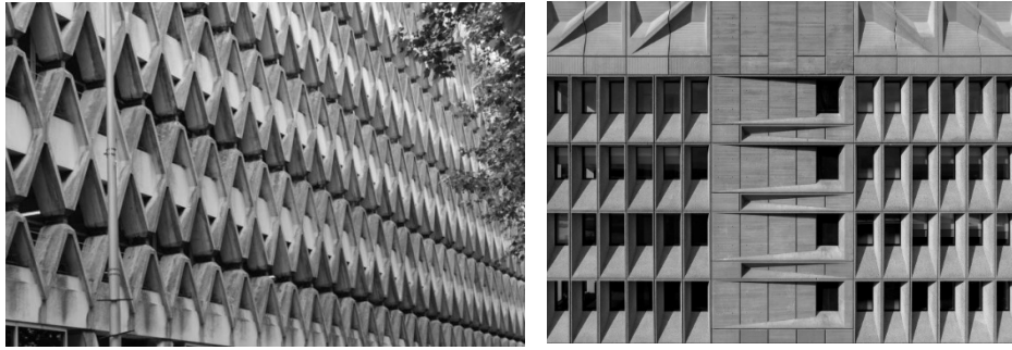
Figure III.VI and Figure III.VII. Precast elements make for a monolithic, rhythmic façade. Sources: Neman, R.; Hommes Studio
