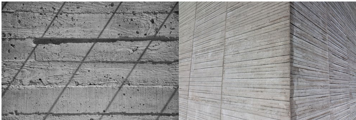
Figure III.I and Figure III.II. Wooden imprint texture on surface concrete. Source: neil mp; Beton Brut
