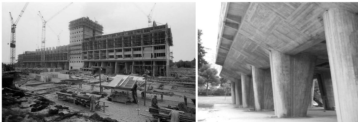
Figure III.III and Figure III.IV. Construction Process and Béton Brut in Unité D’Habitation. Source: Wagner-Conzelmann, S.; Glasgowfoodie
