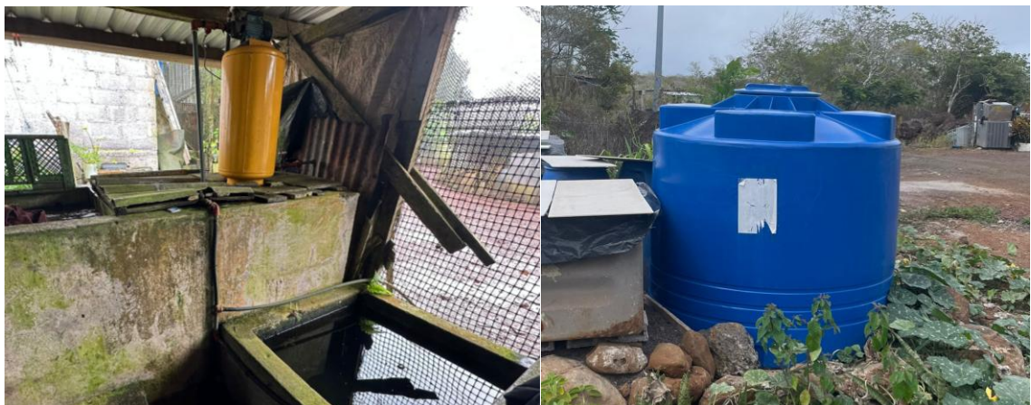
Figure 6: Examples of a cistern (left) and a tank (right)
