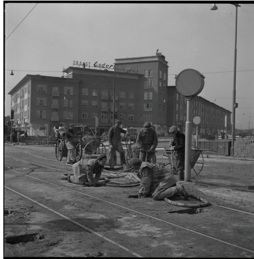
Fig. 12: Construction on the Pleinweg, with the Maastunnelplein in the background on the right. Across the street is the Esders clothing building. (Fototechnische Dienst Rotterdam, 1951)
