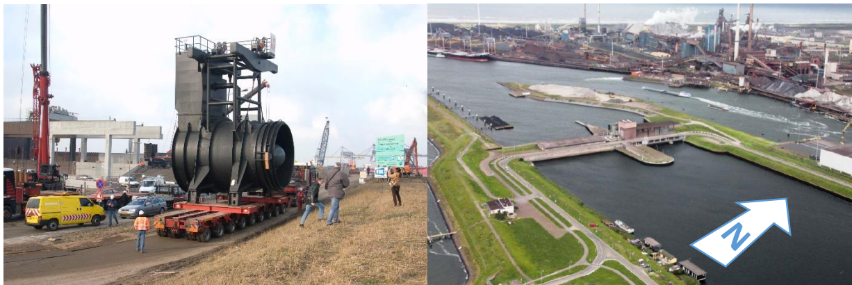
Figure 17 Instalment of the new pump in 2004 (left) and a view of pumping station complex of IJmuiden (right) (beeldbank.rws.nl)
