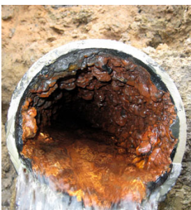
Figure 1.8. Biofilm and deposits in a water pipe. Adapted from: WaterCareer, 2015
