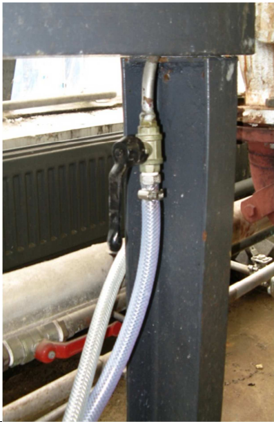
Figure M.15. Air valve for the large belt filter
