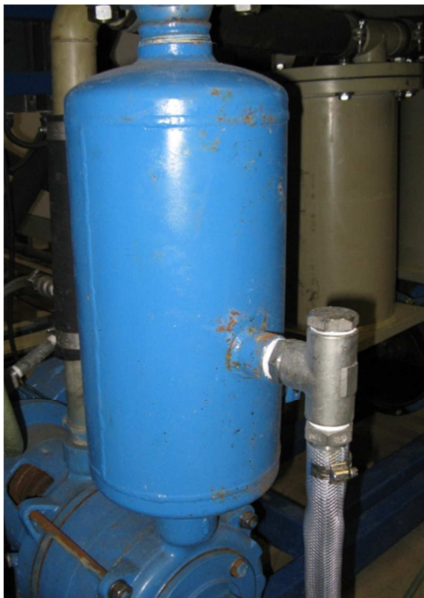
Figure M.22. The separator vessel of the vacuum pump.
