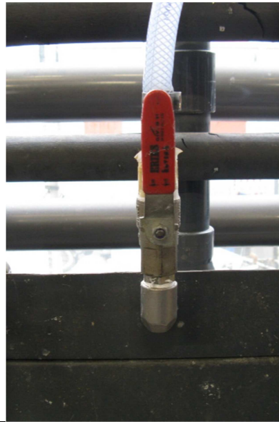
Figure M.16. Water supply to the large belt filter.
