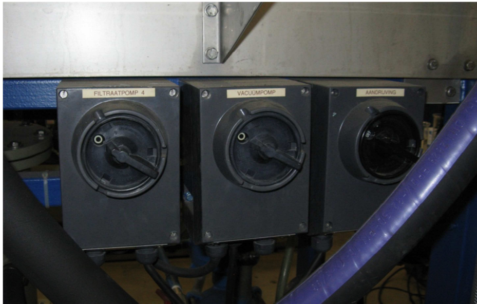
Figure M.18. The black switches at the back of the belt filter. The switches in the photo are used for Filtrate pump 4, the vacuum pump and the belt filter (“Aandrijving”)
