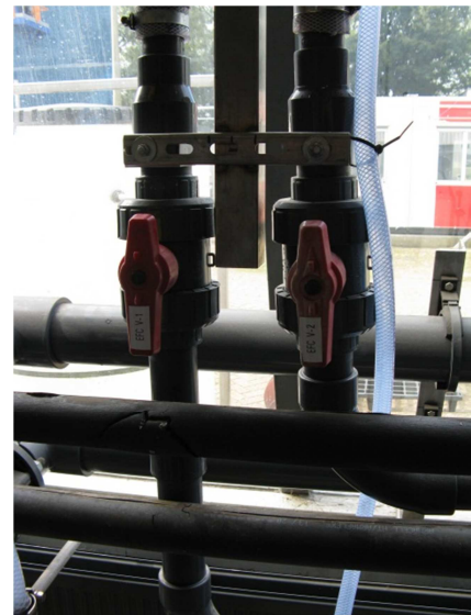
Figure M.3: Cooling water valves (in open position)
