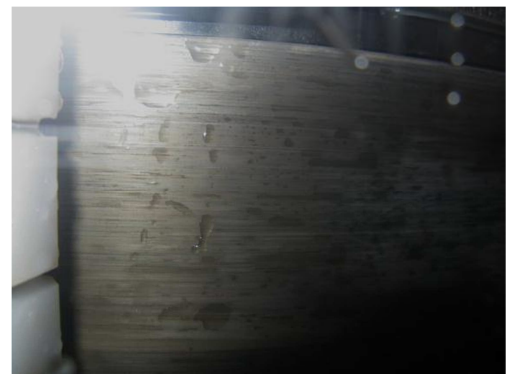
Figure 4.19. After the experiment with the industrial sodium sulfate solution to which NaCl was added the heat exchanger surfaces were found to be covered with a black corrosion layer.
