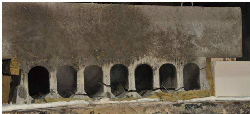
Figure 4-3: Breaking off of webs of hollow core slabs because of shear stresses caused by unequal deformations in lower and upper shell (Source: Cement)
