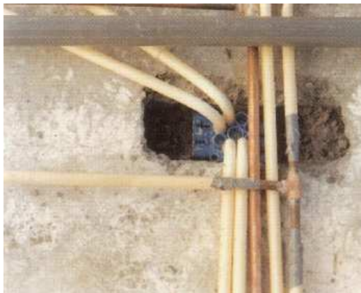
Figure 4-5: Central box (In Dutch: centraaldoos) for wires placed in concrete top layer (Source: Dycore)
