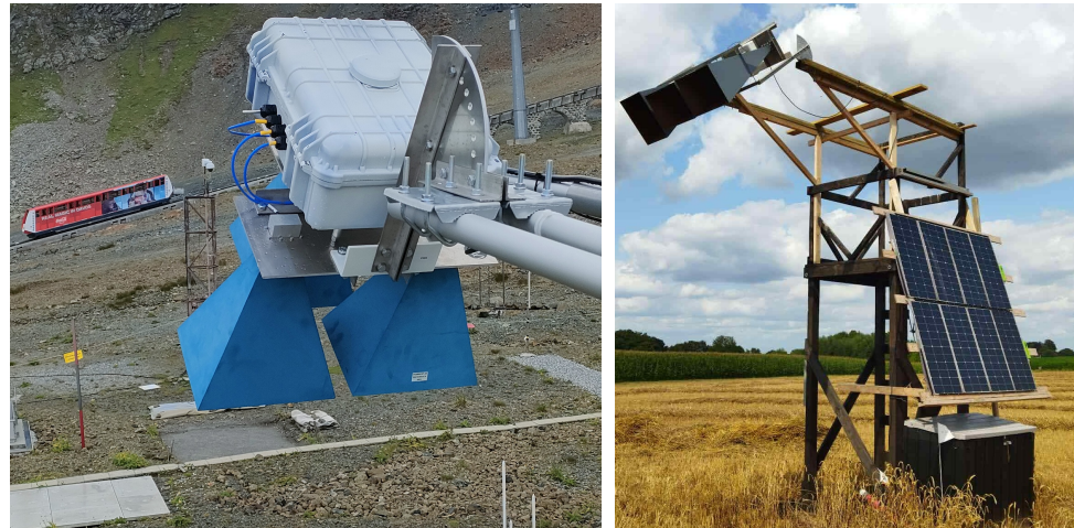
Figure 2. Field installation of the two radar systems showing two potential applications. The left tower, equipped with smaller horn antennas, operates in the C-band and is powered from the grid. The focus of this setup lies in measuring the soil–snow profile. This radar was installed during the summer at Weissfluhjoch, Switzerland, when the site was free of snow. The right tower, located in at Louvain-la-Neuve, Belgium, fitted with larger horn antennas, operates in the L-band and is supplied by a solar-powered battery system. Measurements performed at this location focus on the soil–vegetation profile.
