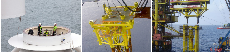
Figure 1.10: Guiding a lifted object during installation jobs; human guidance [l], guiding funnels/holes [m], guiding piles [r]
