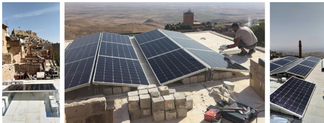
FIG. 9 Photovoltaic panels installed on the flat roof of Tamirevi. Source: KMKD Tamirevi Archives, taken by Süreyya Topaloğlu
