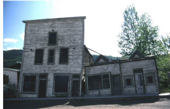
(b) Tilted building due to thawing of underlying permafrost (from National Snow and Ice Data Center)
