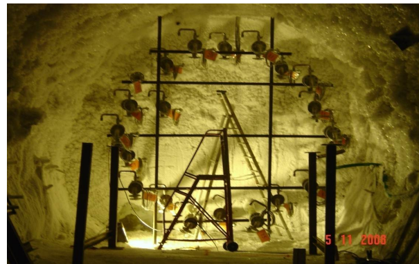
(b) Brine Circulating Pipes at the Face
