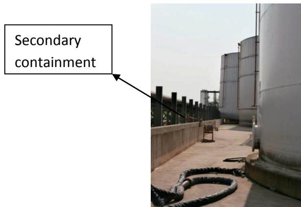
Figure 4-2 Secondary containment around storage tanks, Stolt-Nielsen terminal, New Orleans
