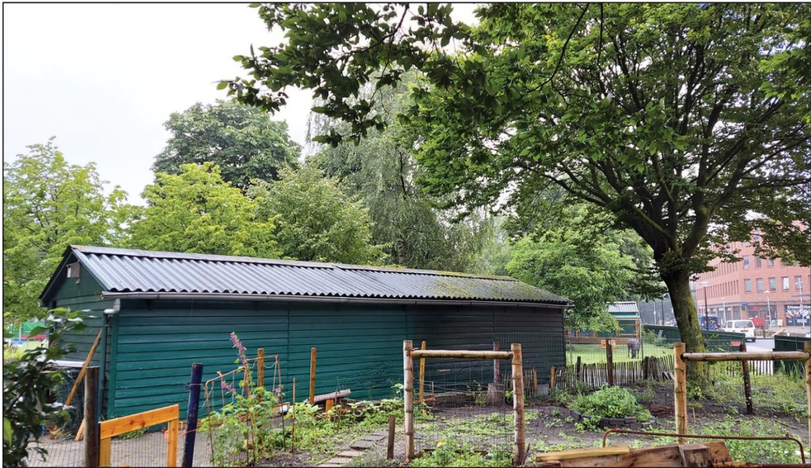
Picture 56: shows the location of site 11, where the exposed roof is partially colonized by living organisms (own picture)
