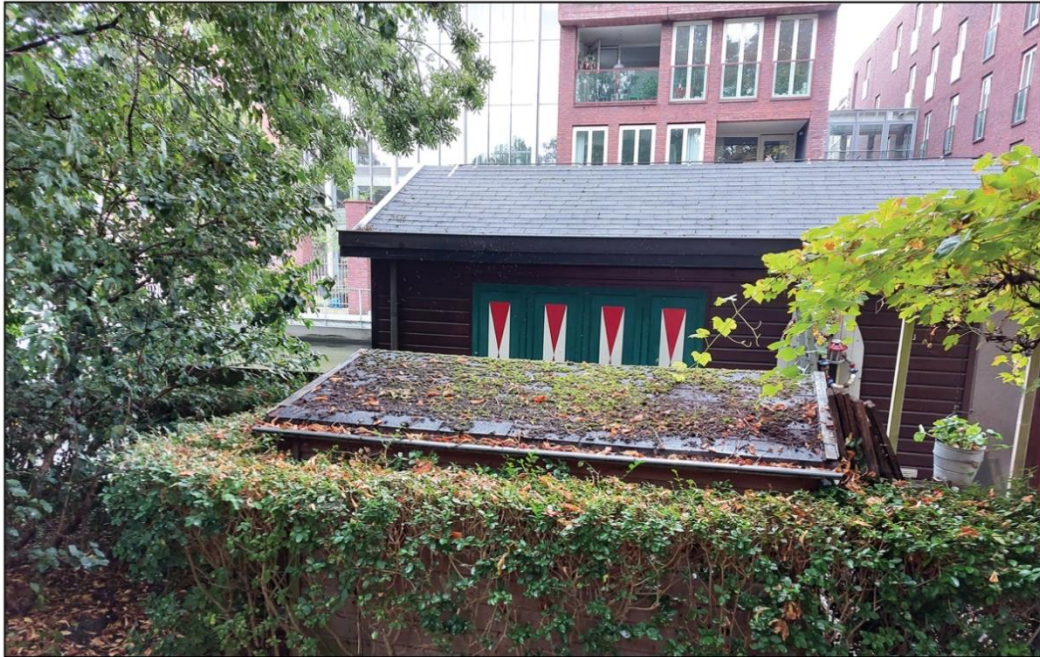
Picture 37: shows the location of site 6, the storage house roof (own picture)
