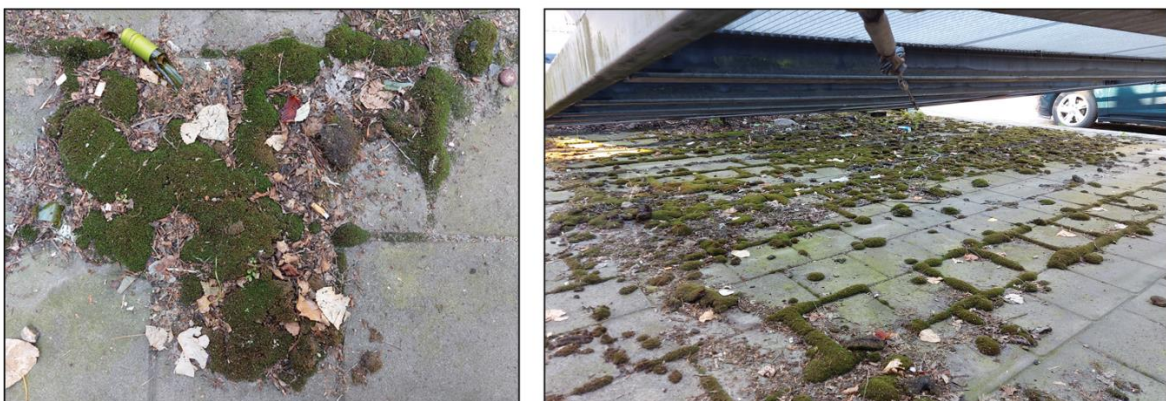
Picture 2: Mosses growing underneath the steel slope bridge (own picture)
