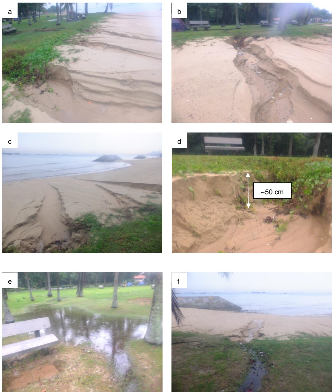
Figure 6.13 Sliding off of upper beach berm during flash floods, East Coast Park. Figures (c) shows the cuts into the beach berm and the path followed during washing out of sediment. In (d) the size of the cut is indicated, being about 50 centimetres deep in all of the cuts. Figures (e) and (f) show the accumulation of rain water above the beach berm, and the flow of this water towards the beach, respectively. The phenomenon was observed in between headlands 8, 9 and 10 on 13 December 2012. No records have been found of similar observations at other locations, yet.
