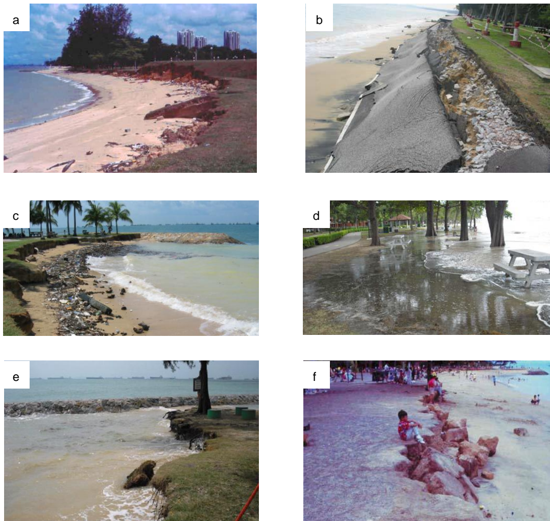
Figure 1.3 Photographs all re-used with permission from Teh Tiong-Sa, professor at the National University of Singapore and researcher at the Tropical Marine Science Institute in Singapore: (a) cliff erosion westward of headland 19, 1992; (b) undermining and failure of path due to berm erosion, 2002; (c) berm erosion in the lee of headland 3, 2004; (d) inundation landward of the high water mark during extreme high tide, 2001; (e) inundation and erosion in the lee of a headland, date and location unknown; (f) scarp retreat near McDonald's, 1991. All photographs were taken along East Coast Park. For the locations of the photos reference is made to Figure 3.7. (source: http://geogallars.com/geo/geoteachers.php )
