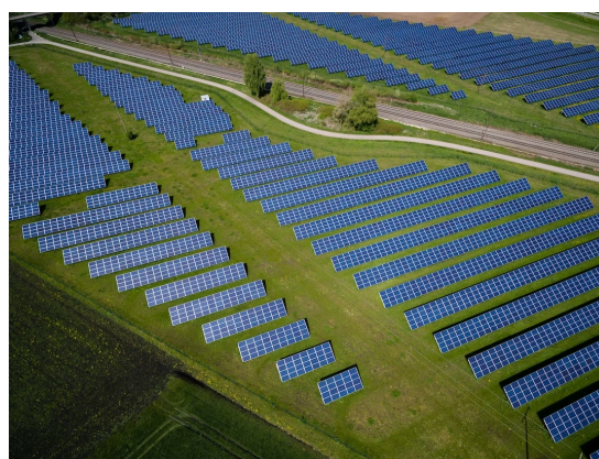
(b) Large scale solar plant.
