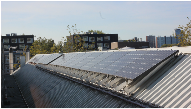
(a) PV panels used for the AC connected ESS experimental setup.
