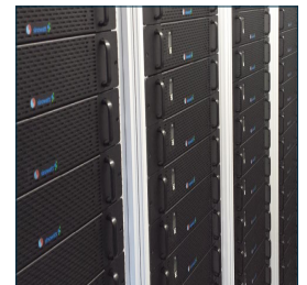
Batteries in 19" racks
