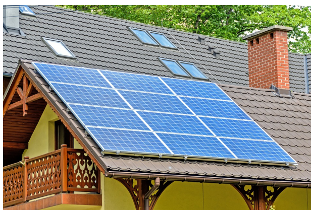
(a) Residential photovoltaic system.
